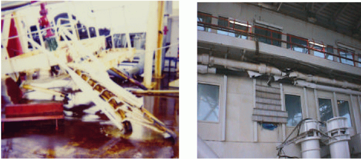
Figure 1.2: Damage to the fire fighting platform of the Emerald FSU (Floating Storage Unit, left) and the damage and first repair of a window after a green water incident on the Varg FPSO (right)
